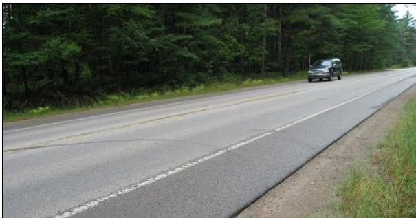
An attached trail might look something like this section of the Boyne City/Charlevoix Road near Young State Park.
